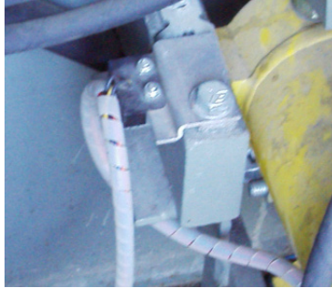
Prox switch mount used before 9/1/2009
